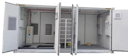
1075KW HH ESS
